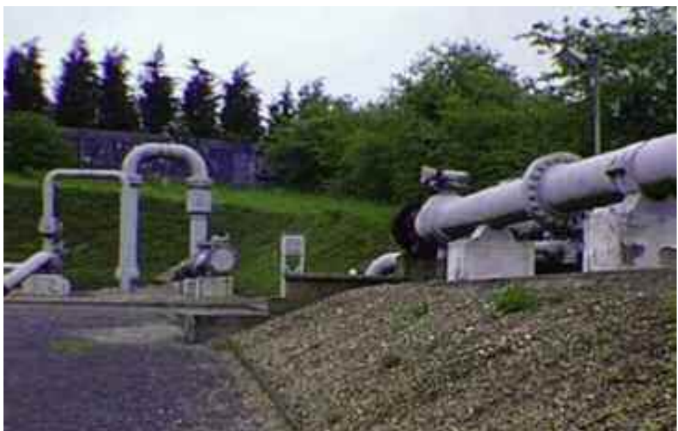
Figure 3 Surface pipelines within an oil fuel depot
